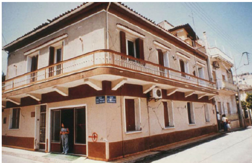
Fig. 16.8 Unreinforced masonry with RC floors, grade of damage 3, in Greece 1995 (Grünthal 1998, EMS-98 scale)
