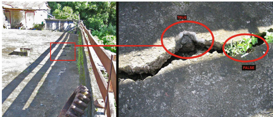
Fig. 16.6 False declaration by the inhabitants of terrace collapse (Les Saintes earthquake 2004). In fact the terrace is not collapse and it's only an increase of existing crack created by an amplification of differential collapse. We can see on the right picture the presence of vegetation in the crack, meaning the age of this damage
